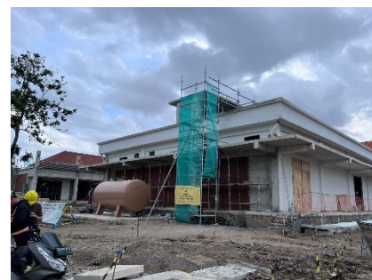
We are shown from the progress of the ground water tank project. Later, the processed GWT will be recycled and distributed back to the area around the SEZ
