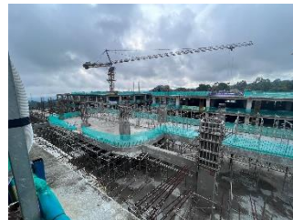
PTPP builds Manik Mas building, which will be used as a vehicle parking facility.
